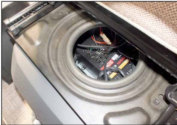
Battery charger underneath the driver seat (sample illustration)
