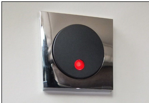
Switch for the waste water tank heating on the seat box
