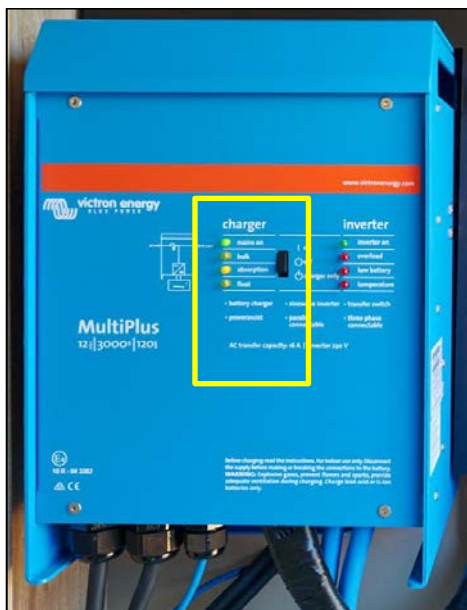
Battery charger in the rear garage (sample illustration)
