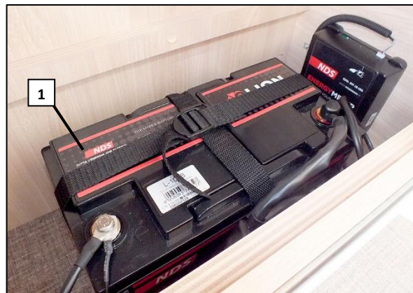
Living room battery in the bed box, left (sample illustration)
