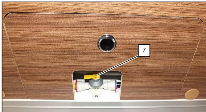
Yellow drain valve for the Alde hot water heating
