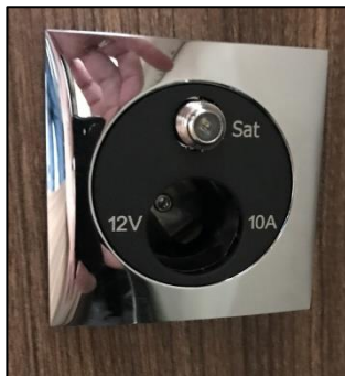
TV connection (interior)
