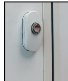
Service hatch latched but not locked (the cylinder protrudes).
