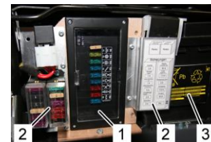
12 V fuse box
