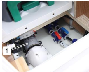
Water pump with drain cocks
