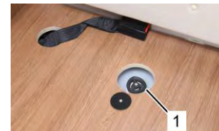
Drain cock fresh water tank
