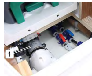
Drain cocks pipe system
