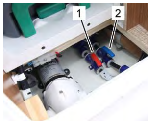
Drain cocks pipe system
