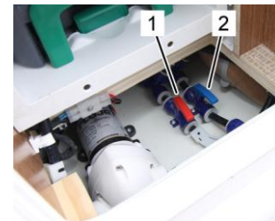
Drain cocks pipe system
