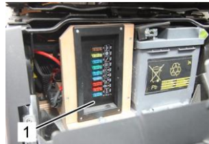
12 V fuse box
