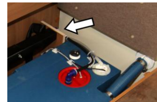
Location of pressure control valve
