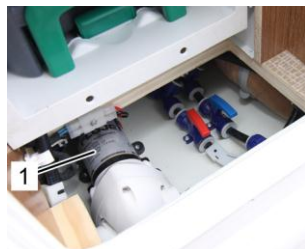
Drain cocks pipe system
