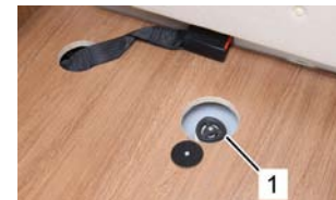
Drain cock fresh water tank
