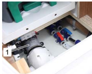
Drain cocks pipe system
