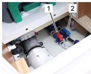
Drain cocks pipe system
