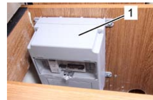
Automatic circuit-breaker 230V
