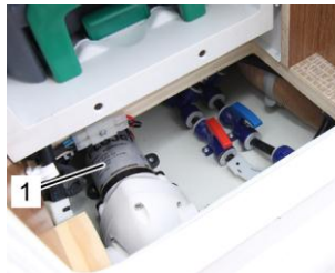
Drain cocks line system
