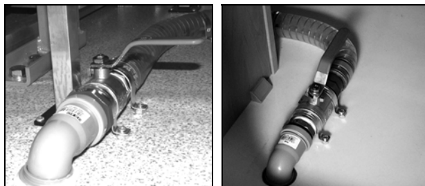
Valve for draining wastewater, closed/open
