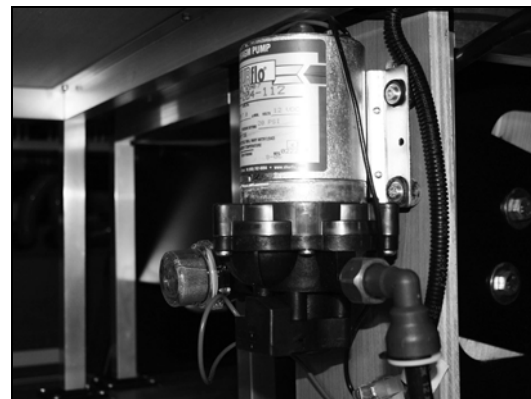
Position of the water pump on your motorhome:
