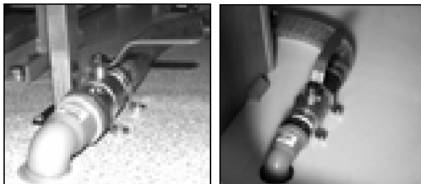
Valve for draining wastewater, closed/open
