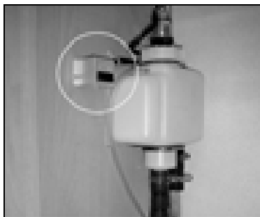
Switch for the 230 V circulation pump
