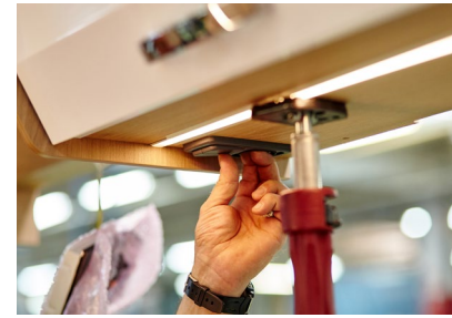
Check of operation and correct installation of the electrical systems.
