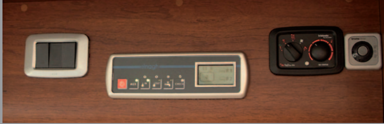
Central control console with LCD screen. Interior and exterior temperature sensors.
